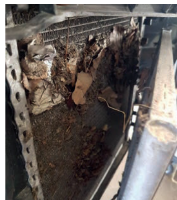
Dirt build-up between radiator and condenser
